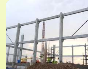
UPL Warehouse, Raipur
