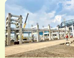
Deepak Chem Tech Ltd., Gujarat
